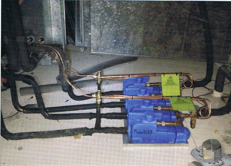
Installation of two XDX valves on each stage of a two-stage package unit, with insulating jackets.
